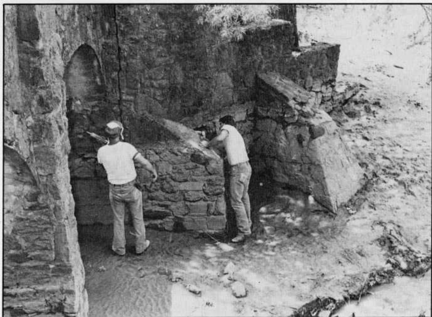
Tuckpointers from the OU physical plant, Stan Airington, left, and Ron Kinnard, turn volunteer stone masons on weekends to repair the stonework on the bridges, much of which has been stripped away by cracks in the concrete and erosion.
