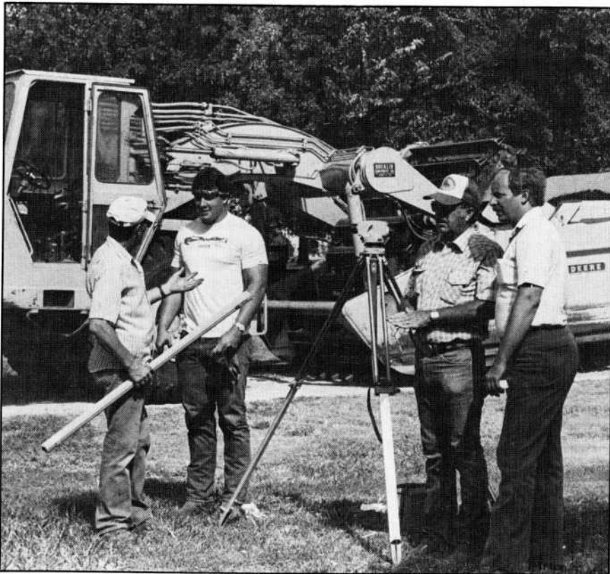
While his equipment operators, Roy Anderson, left, and Travis Simpson, get their assignments straight, Theron Simpson of Coot Simpson Construction Co., second from right with OUPD Lt. Richard Hamilton, prepares to shoot the elevation for terracing along the edge of the channel which they have just dug to create the new duck island. In real life, Travis is a member of the Big Red offensive line.
