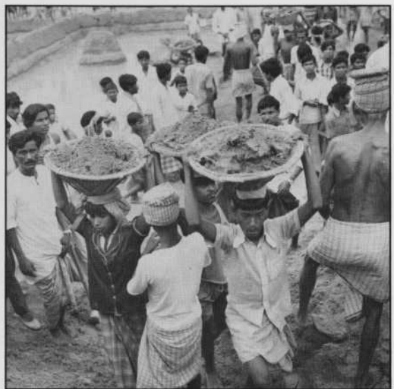
In this close-up, workers are shown carrying earth to the embankment in their headbaskets. The monsoon rains stand in the area in the background where the earth has been removed. The pyramid-shaped measuring device in the water is used by the gang chiefs to monitor work achievements.
