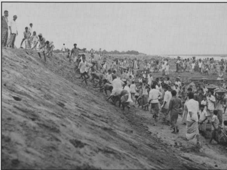
Desperate to secure enough food to feed their families, approximately 735,000 rural, landless laborers in this country alone participated in 1975 Food for Relief Work projects, building flood control embankments such as the one pictured above. Using primitive headbaskets and hoes, they swarm over the work site to dig up the earth which will earn them approximately 60,000 metric tons of wheat.
