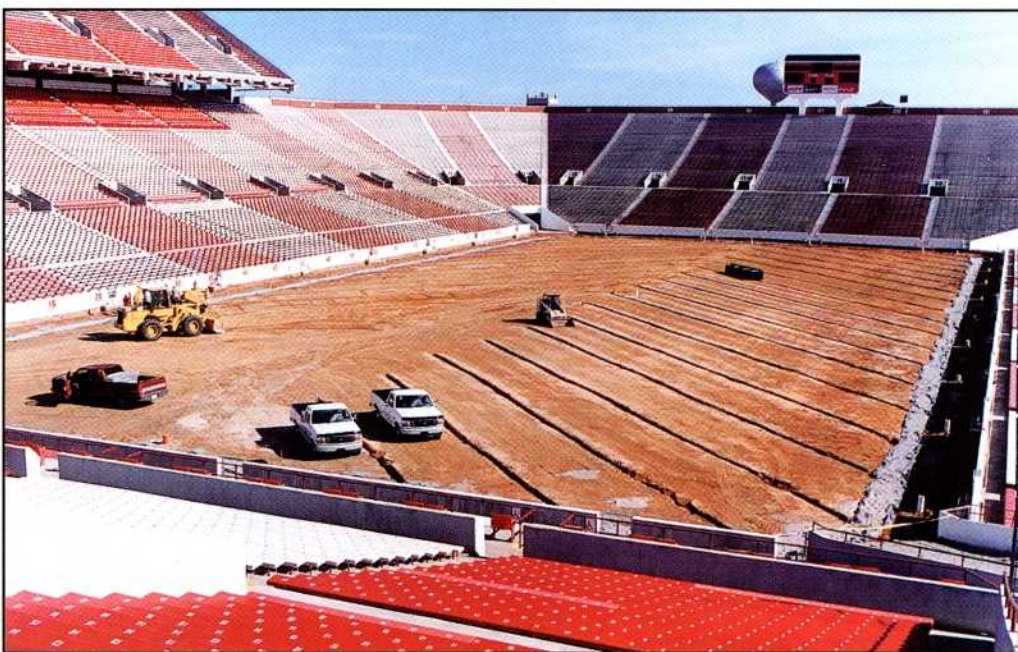
The gravity-based sub-drainage system consists of V-shaped rows of plastic, gravel-filled pipes leading to drains that can remove 10-to-12 inches of rain an hour from the field.
