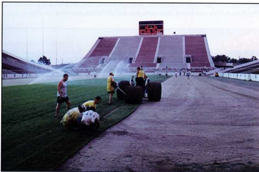
The ground crew manually wrestles the 50-foot-long rolls of turf into place as the sprinklers apply an immediate soaking. The surface was covered in 48 hours.
