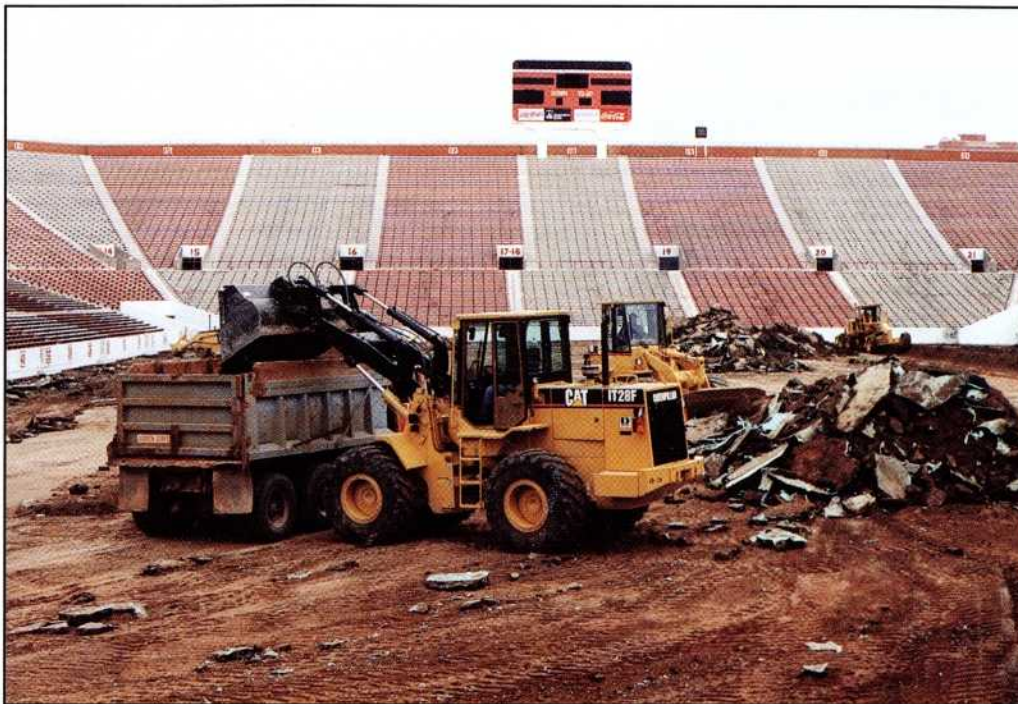
Heavy equipment is called in to break up and remove the old asphalt base, which was nearly six inches thick. Truckload after truckload then were hauled out of the stadium.
