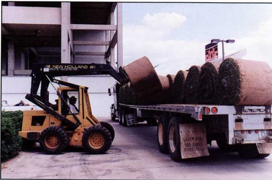
A specially constructed tractor unloads the Tifway 419 Bermuda that just hours earlier had been cut and rolled at a sod farm near Tulsa. Bundled in 30-inch-by-50-foot rolls, the grass had to be in place on the growing zone within hours of being cut.
