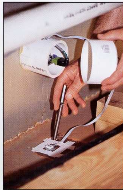
OU engineers attach a motion sensor called an accelerometer to a bridge beam at the Purcell test site.
