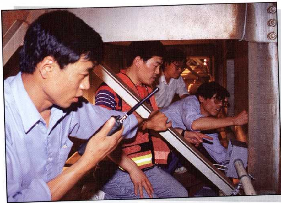
International student engineers working under the bridge to pull wire through a conduit are, from left, L. Liu, C. Mo, Q. He and S. Sha.
