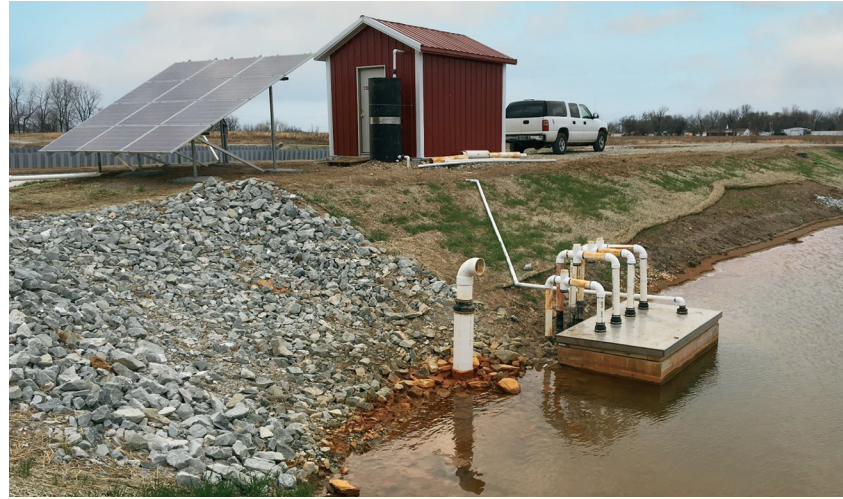
Nairn and students designed and built a custom solar system to power the passive treatment at the Southeast Commerce site. Energy from the solar panels is stored in batteries inside the shed. The batteries power blowers that force air into aerators in the treatment ponds, oxygenating the water.
