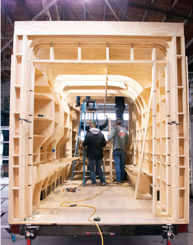
Construction science students in OU's "Design + Build" class assemble the mobile unit, which was built from donated materials.
