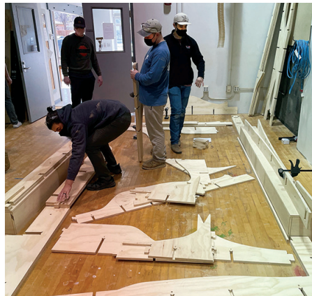
The interior of the mobile medical unit was designed for ease of construction as a machine-milled "kit of parts." Builders only need a few simple tools, like a drill and rubber mallet.
