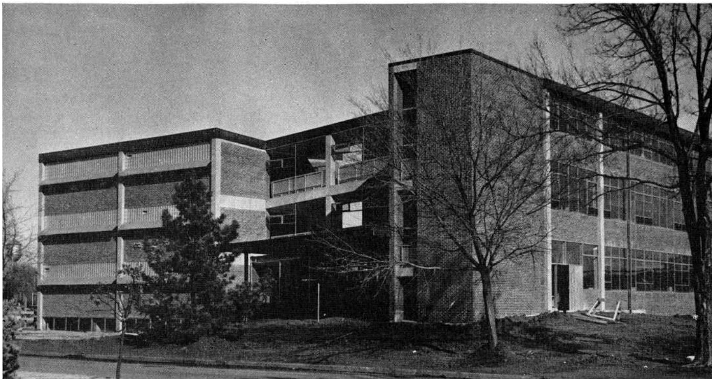
Almost ready for occupancy, this structure is the first two units of the Geology and Mineral Industries building which the School of Geology will occupy as its new home in the near future. Ground already has been broken for two additional units of the building.
