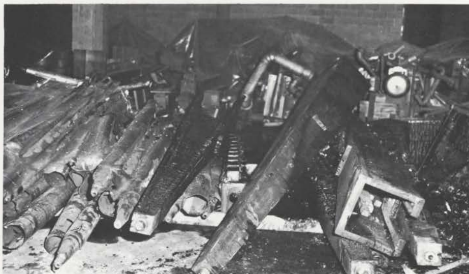
DAMAGED PIPEWORK clearly shows in this dramatic photo of a wanton attempt at purposeless destruction.
