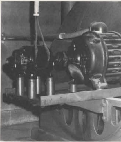
The 15 volt, 22 ampere generator runs from the driveshaft of 15 hp 440 volt 3 phase Woods motor. The Orgoblo (right) generates 10 and 15 inch pressures. Blower room is off the right chamber.
