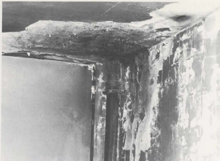
Damage to ceiling and wall of right chamber caused by years of water seepage from a leaky roof. Luckily, no irreparable damage resulted.
