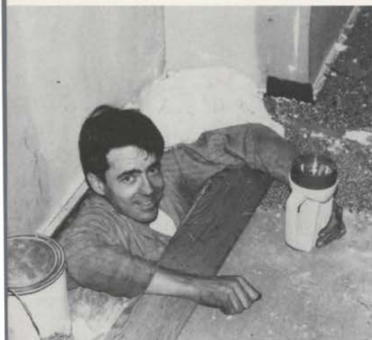
They even came out of the woodwork! Leo, the Cable Saver, had the dirty task of crawling through a small hole to save the console cable. It finally disappeared beneath floor joists, couldn't be pulled loose and had to be cut. (George Brown Photo)
