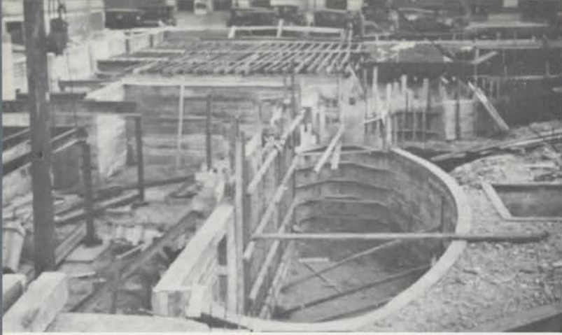
Many hundreds of musicians have been hoisted into view on the orchestra lift being formed here. Dressing rooms are beneath stage to left.
