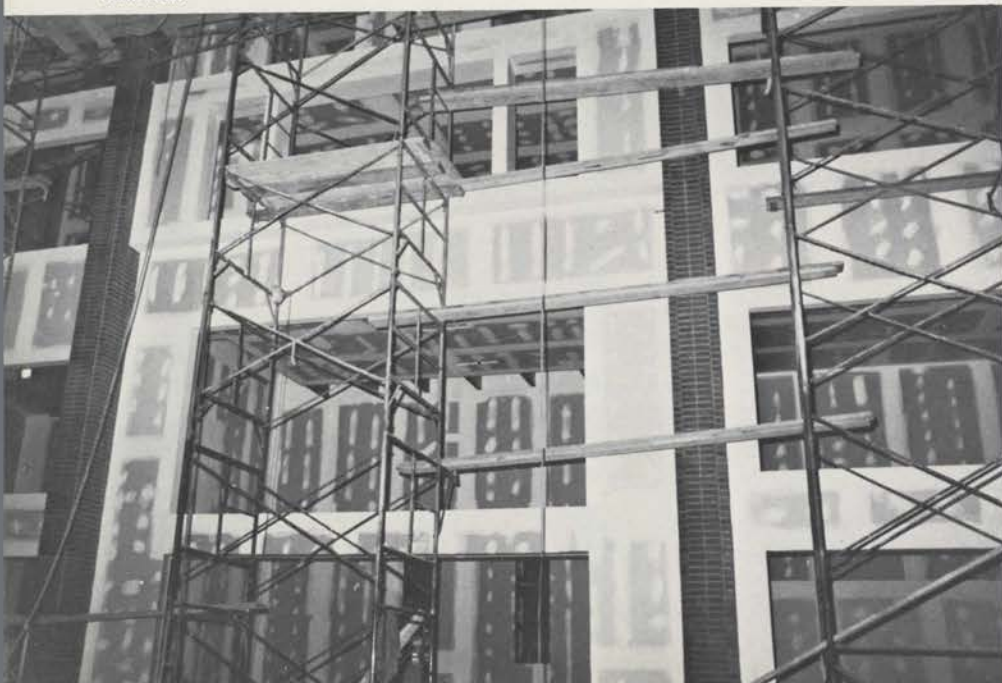
Behind the scaffolding, work nears completion on the expression chambers that will cover one wall of Wurlitzer Hall.
