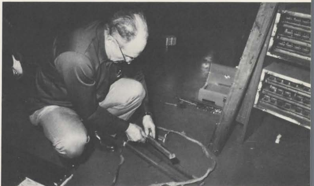
Lou Rosa, friend and confidant to the late Fanny Wurlitzer, is still an active member of the Wurlitzer staff. Here he checks the relay wiring on The Mightiest Wurlitzer during installation at Wurlitzer Corporate Headquarters in DeKalb, IL.
