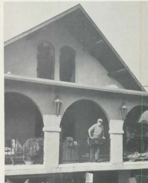
Ray Ledwon, John's dad, awaits the forklift which will lower the console (right niche) to ground level then take it down the steep driveway to the flatbed truck.
