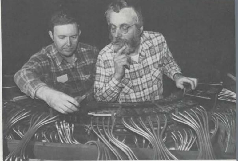
Tim Johnson (left) and Bill Snyder looking over the new contact blocks before installing the top rail. (Photo by Dave Carter)
