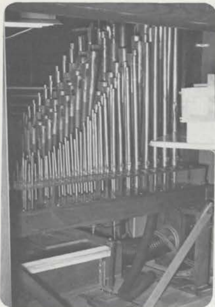
Partial chamber view showing shutter motors on right. (F.R. Gandy photo)
