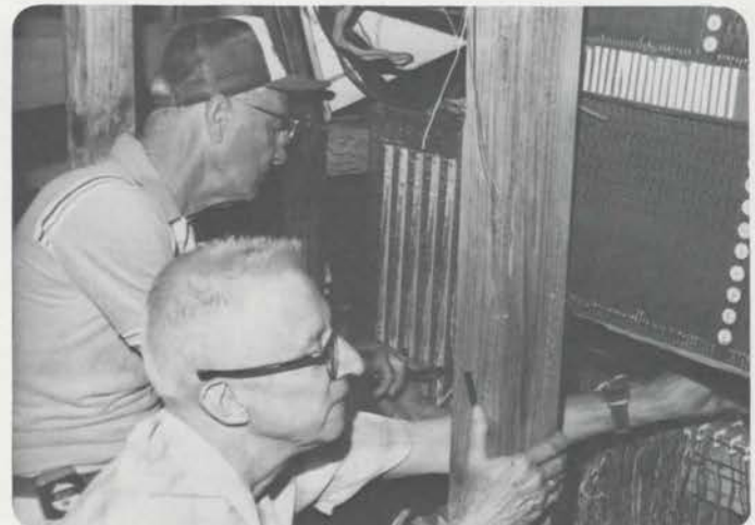
Lee Wilson, rear, and Ed Lawrence checking the wiring and solid-state units in the console of the 3/12 Wurlitzer which CFTOS is installing in the Tampa Theatre. (John Otterson photo)
