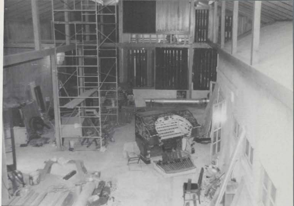
San Francisco Fox Theatre 4/36 Wurlitzer being installed in the Lanterman home, circa 1967.
