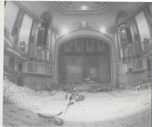
Interior demolition (August 1973) as the theatre is converted for multiple screen operation.
