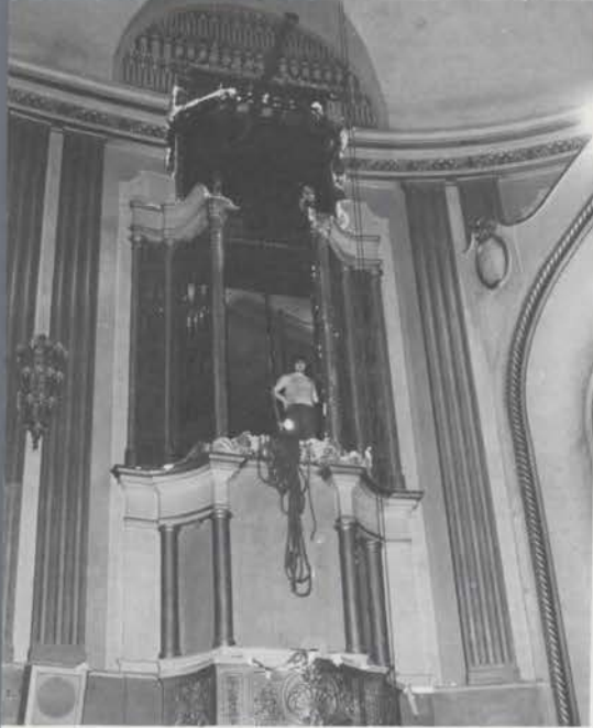
Front of the Main chamber after removal completed, showing steel beam attached to the theatre structure for the necessary block and tackle.
