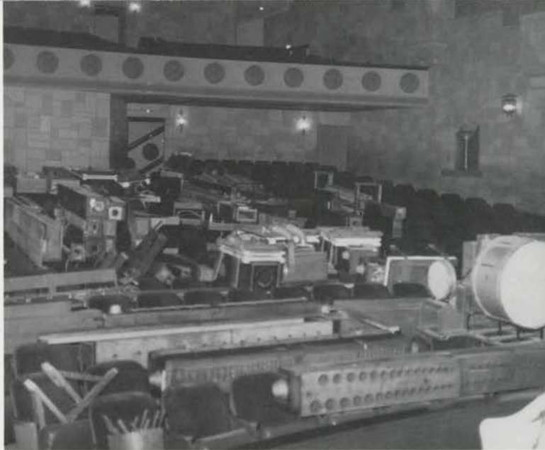
Chests, reservoirs, percussions and pipework are stacked across Granada Theatre seats awaiting installation in chambers formerly occupied by a Robert-Morton organ. The incoming Barton has been leased for 20 years from Kansas City Theatre Organ, Inc. It will be increased from 11 to 20 ranks.
