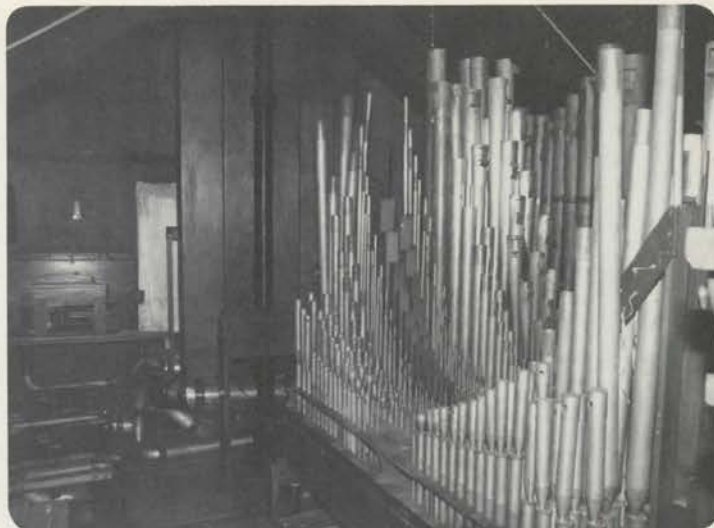
Attic chamber of Paul Wasserman's home installation. (TATOS photo)
