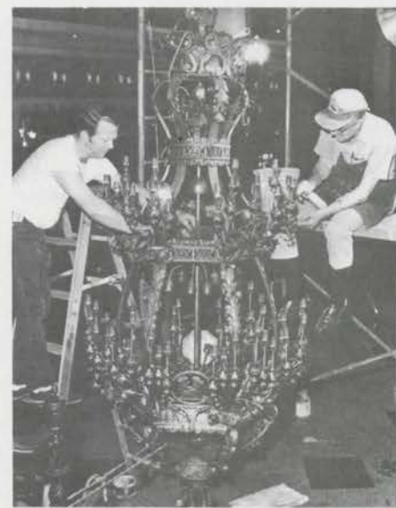
Richard Parker and Bob Johnson complete re-wiring of the main chandelier in the grand lobby of The Alabama Theatre. Each broken piece of glass was exactly duplicated and every wire was replaced.
