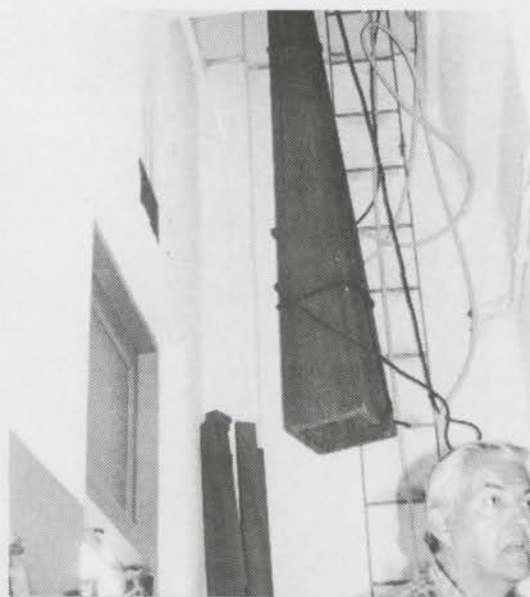
Frank Way supervising the hoisting of the 16' extension pipes up through the chamber access — a 3' x 4' trap door. (Even the seven-rank chest went through [!] with an inch to spare!
