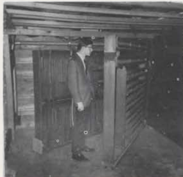
Relay in roll-out position (note the casters).
