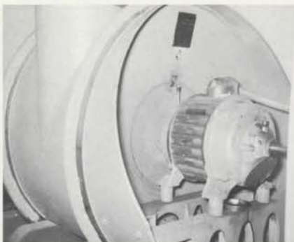
This 10 horsepower motor rotates the "Orgoblo" fan blades. Note the sleeve bearing and associated oil cup, also the oil cup at the other end of the motor shaft. Keeping them full saves burnouts.
