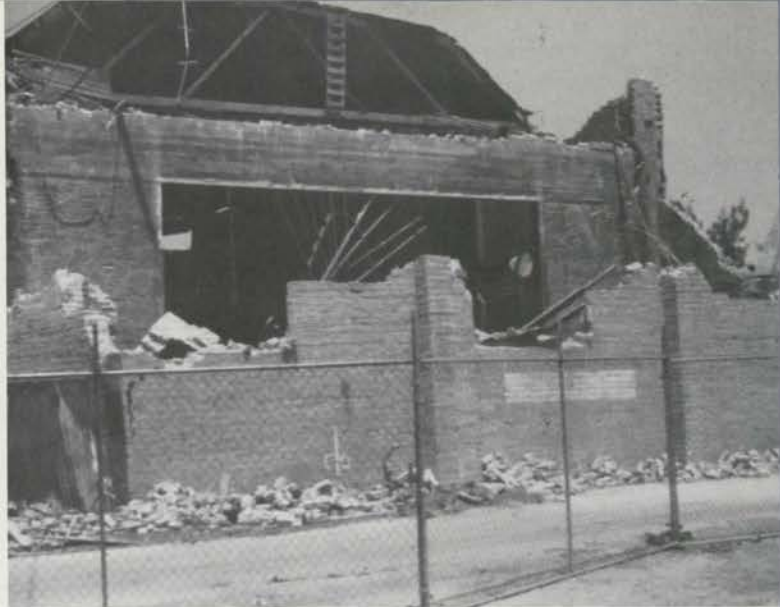
Rear view of the State Theatre, Coalinga, California, showing the stage house collapsed but the concrete proscenium arch still standing. (DeLay photo)
