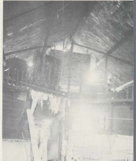
Light leaks through the ruined Percussion Chamber (above). A large wind chest (foreground), removed from behind the charred swell shutters, awaits transportation.
