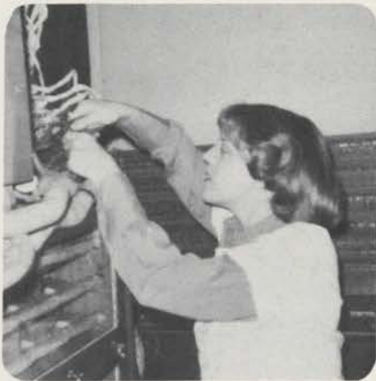
Sonia Carlson, wiring piano switch at the relay, Fargo Theatre.
