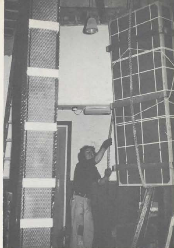
One of the rebuilt manual chests going up through the chamber floor. The new steel work on the left was part of the chamber reinforcing structure that was needed.
