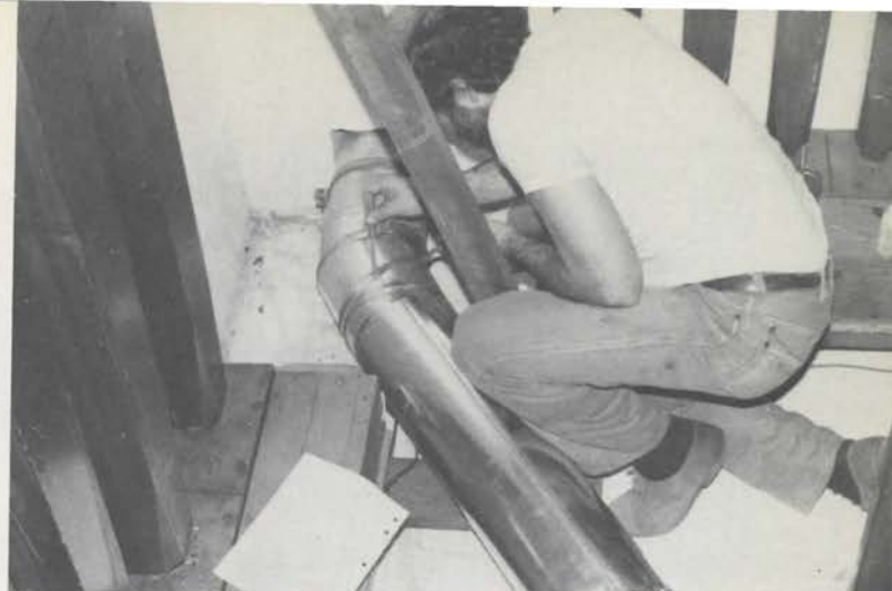
Installing a pipe organ requires many skills. Here Bob solders joints in a new tin wind line.
