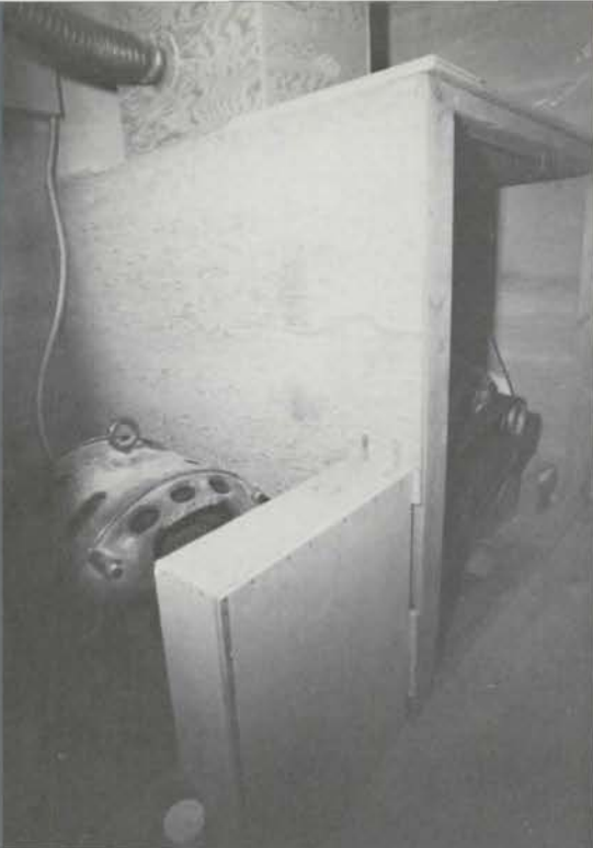
Two-phase motor on left drives blower motor on right with V-belts.
