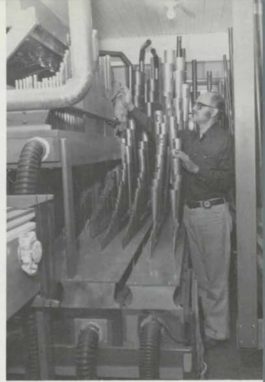
Lance working on the 2/7 hybrid organ in his home in Dilworth. The pipe chamber occupies the front sleeping porch.
