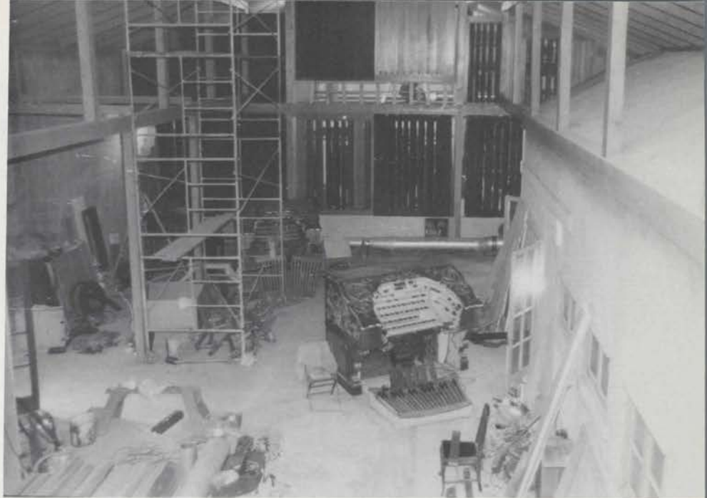
San Francisco Fox Theatre 4/36 Wurlitzer being installed in the Lanterman home, circa 1967.
