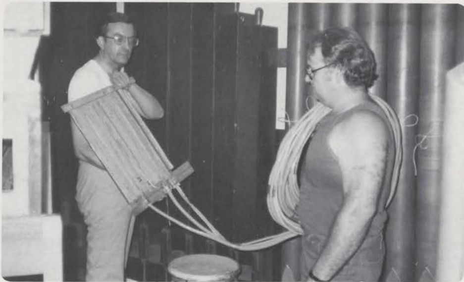
Middletown, New York, Paramount crew members Bob Welch (left) and Bob Seeley prepare to install junction board and cable for the main chamber.
