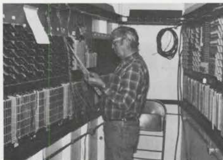
Don Newswanger in the refurbished relay room at Manual High School.
