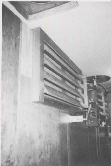
Two swell shades, each measuring two by four feet, are mounted at ceiling height in the narrow chamber space. Both pipe and electronic ranks play at full volume and volume is controlled through the two sets of shades.
