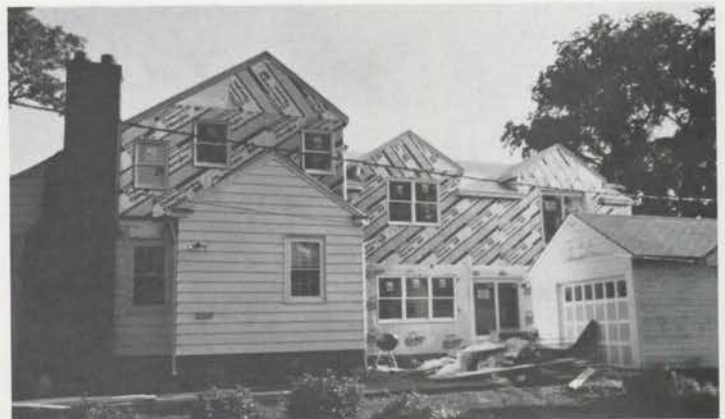
BOB ARNDT'S new music room, which will house his new Arndt "Hope-Jones Unit Orchestra," is only part of the new construction pictured above. The second story blossomed out larger than the first floor.
