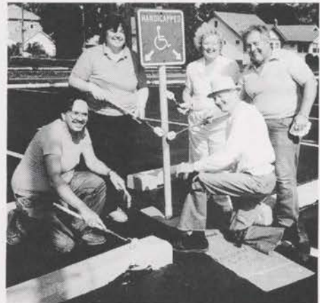
Motor City Roller Derby. David and Michelle Ambory, Dorothy and Ray VanSteenkiste and Jim Green (kneeling, right) managed to go through four gallons of yellow paint to brighten the bumpers and poles in the Redford Theatre parking lot. After resurfacing last year, another sealer was applied and the lots professionally striped. The sign does not apply to any of those pictured. Gil Francis Photo
