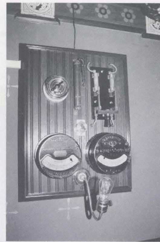
Organ control panel in Gothic library. Antique meters register voltage and amps from organ's DC generator.
