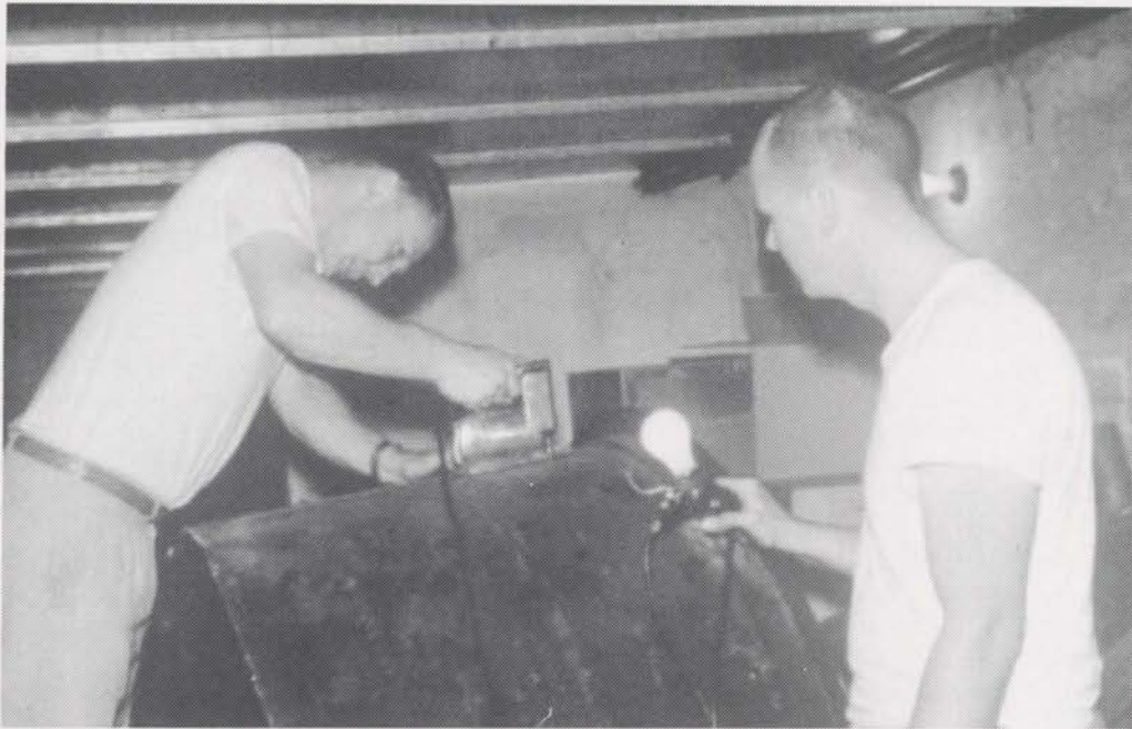
Ron Downer is forced to cut the blower housing to get it through a door. Theatre owners refused to allow the door to be removed.
