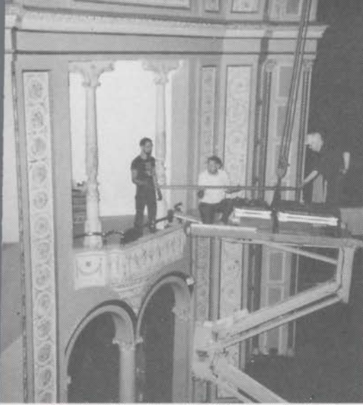
Bardavon (Poughkeepsie, NY) crew members Bruce Audretsch, John Vanderlee and Barb Penrose moving regulators into chambers high above the orchestra. The original 2/7 Wurlitzer is being re-installed. Michael Pruyn photo
