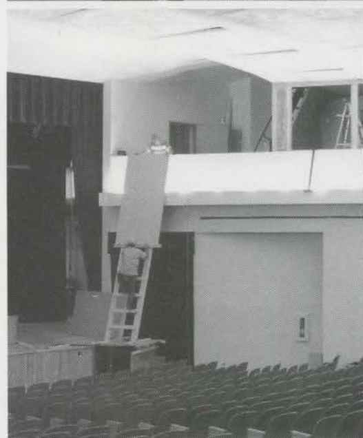
Jim Becker and crew from Castle Contracting worked through the entire Christmas holiday season to complete the pipe chambers.
