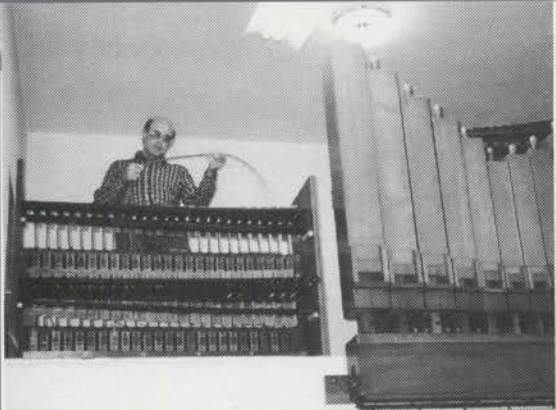
Bob Raymond, Jr. connects cable to the chrysglott in the Ben Hall Wurlitzer at the Lafayette Theatre in Suffern, New York.
