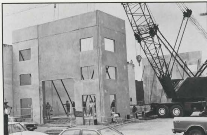
THREE STORIES FOR ORGAN PROJECT —This is the beginning of a 12,600-square-foot pipe organ production palace that adjoins the former Bob White Theatre in Portland, Oregon. It is a real fantasy for its owner Dale M. Haskins.
