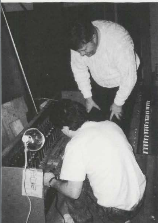
Vern Betourne (top) and Tom Norvell stripping off old wire on percussions.
