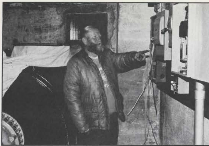
Dale Haskins points out new electric panel boxes installed to handle organ blower motors in the Bob White Theatre building.
