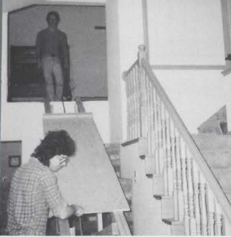
Chests and relay were slid upstairs on this ramp and rail arrangement through the swell shade opening.
