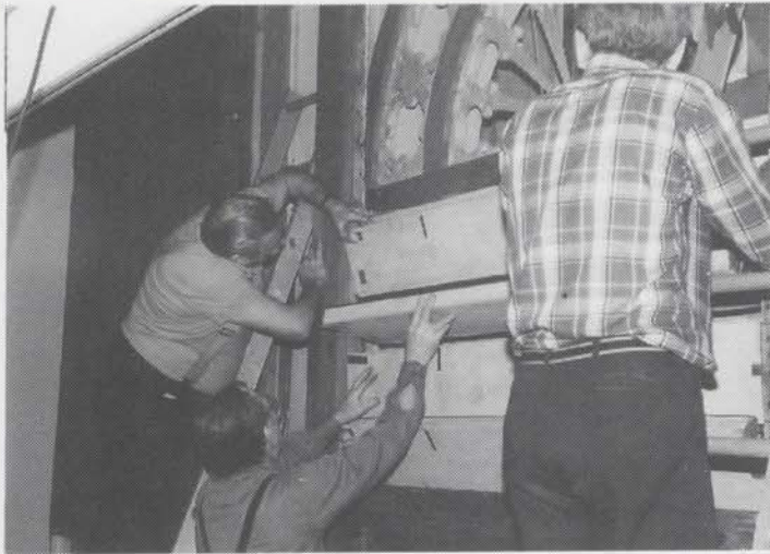
Roy Wilds, Don Johnson, and Bob Scholer (rear view) install shutters behind the grille work.
