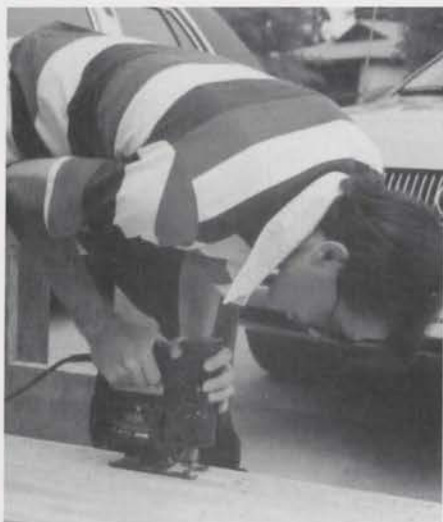
OATOS President Wayne Tilschner, cutting out one of the sixteen openings on the wind trunks for the regulators.
