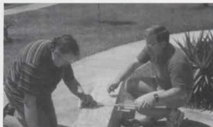
Ted Campbell and OATOS Vice President Ron Bower work on the construction of the wind trunks for the main and solo chambers.
