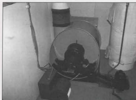
Blower-Generator-Converter in utility room across hall from organ chamber.
