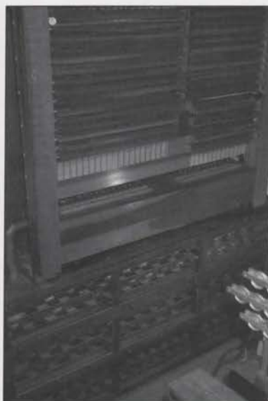
Relay - Spreader Board behind.
