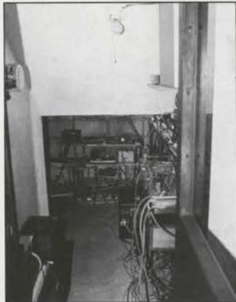
The relay room at Kernal's Korner is crowded.
