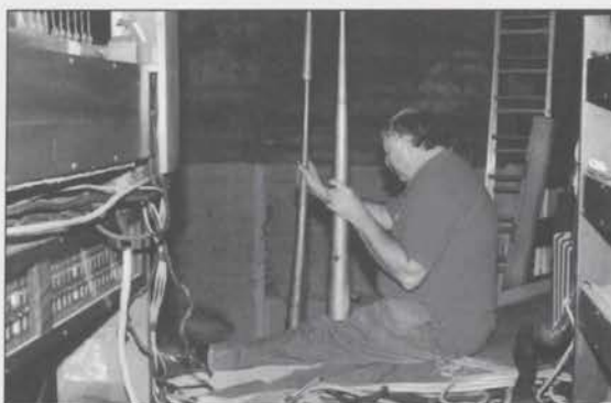
Jim Riley on the relay platform outside the Solo Chamber.
