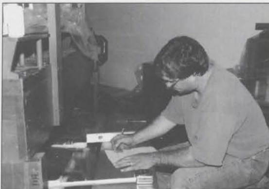
Tom DeLay attempting to engineer the installation of the Vibraphone. It cleared the ceiling with 1-1/2" to spare. Sometimes you get lucky ...
