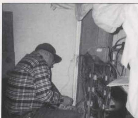
Bill Montague, our telephone engineering expert, wiring the electronic capture system in the console. Don White photo
