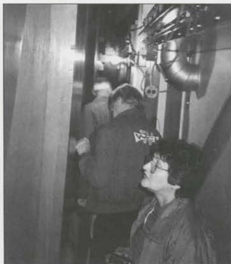
Atlantic City organ crawl -- members make their way through the maze of pipes in the Midmer-Losh chambers.
