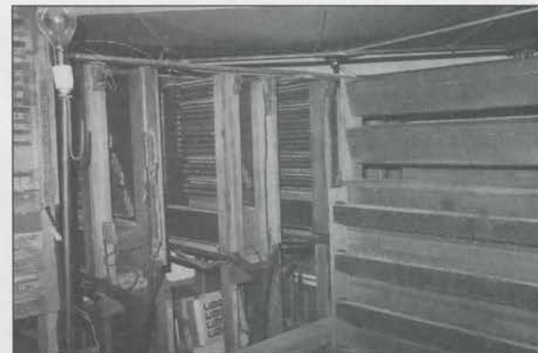
Detroit Fox Relay Room.
