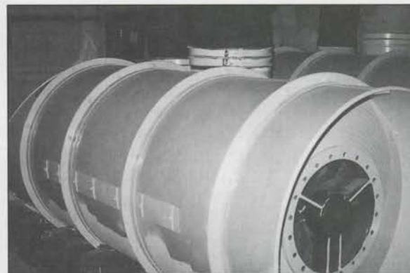
The twin 50 horse power Spencer Orgoblo units.
